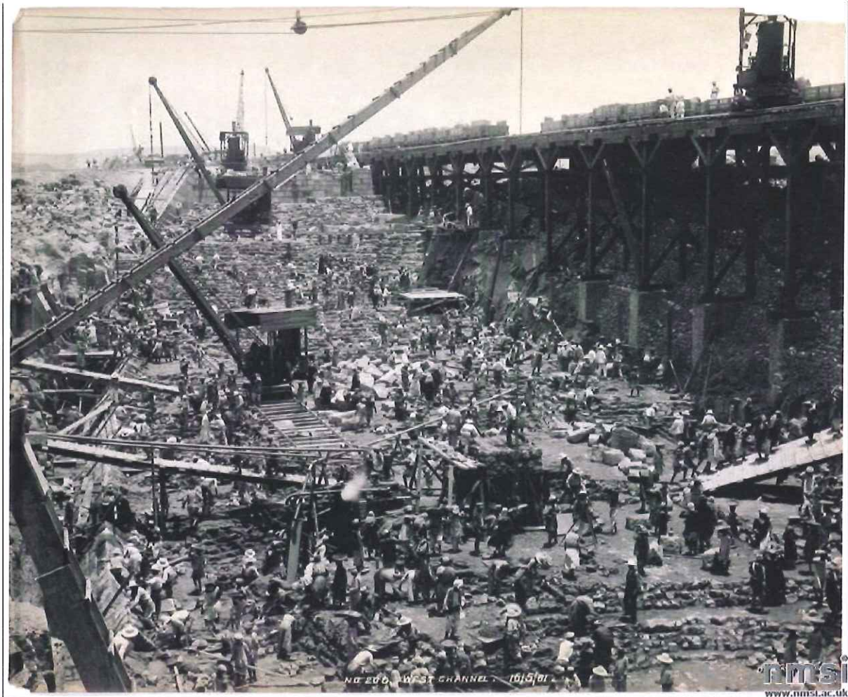
Figure 6 photograph. (200) Central Channel sluices. From North West. [Aswan Dam under construction] / by D. S. George, 16/5/[19]01, signed b.r. and titled.
